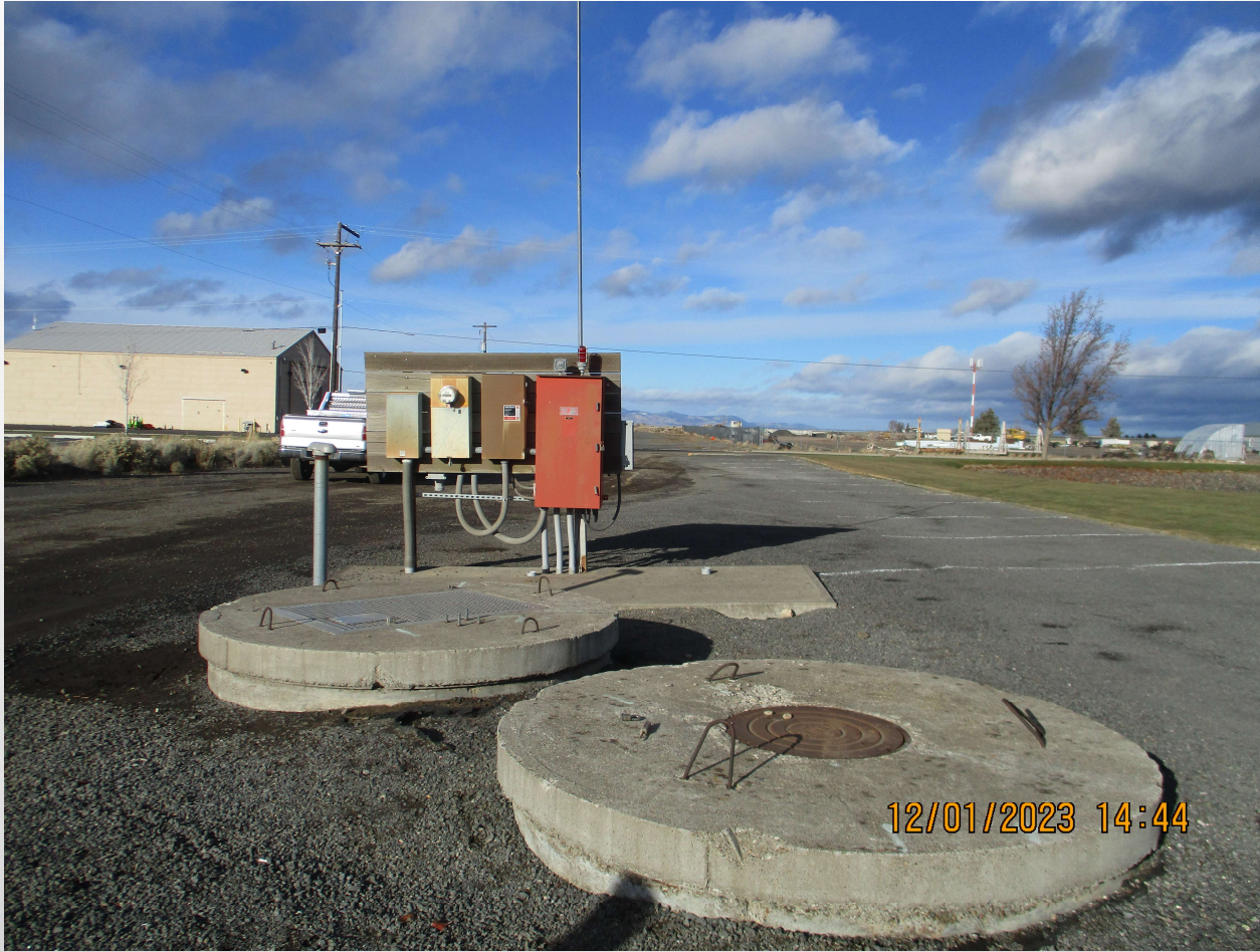
Demers lift station
