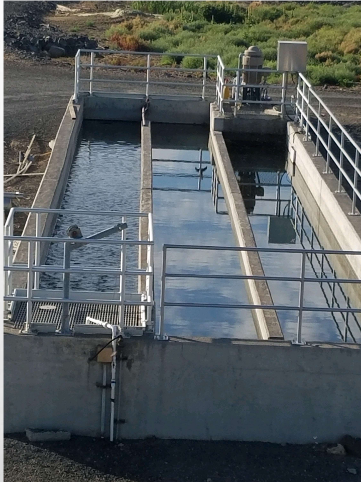
North plant chlorine contact chamber
