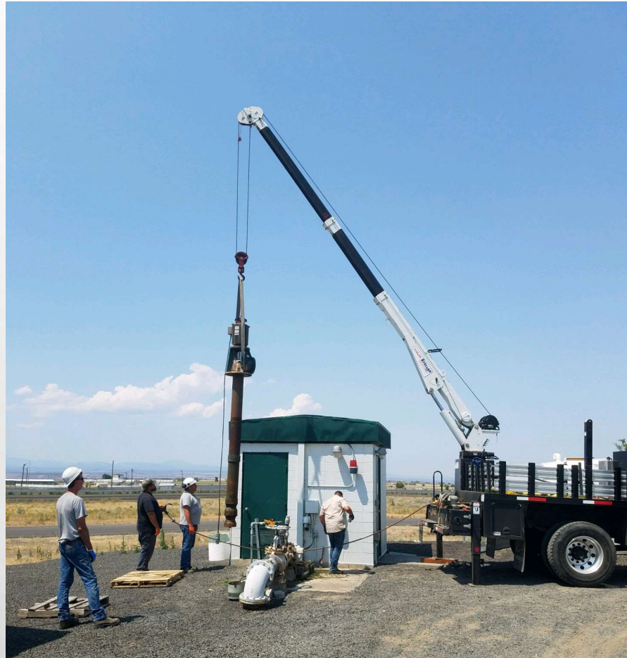
North plant intermediate pump
