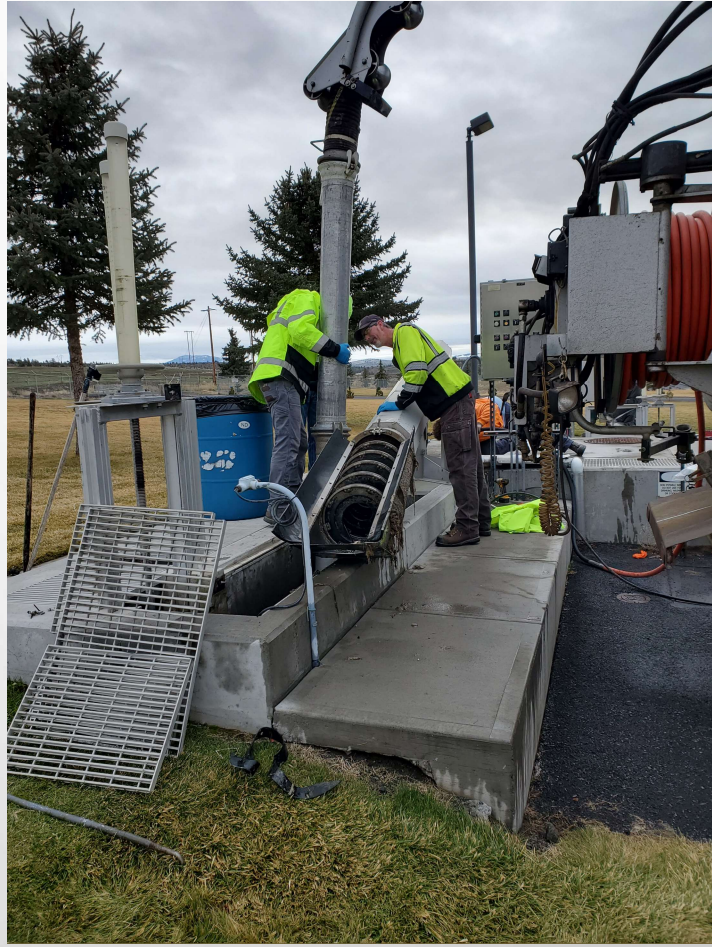
South Plant head works (heliclean)
