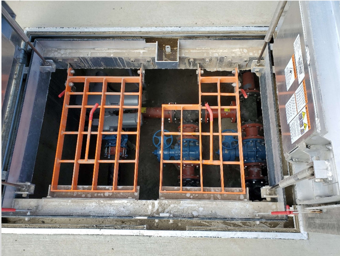
Lift station discharge valves
