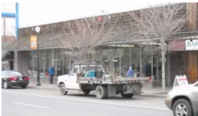
Existing buildings with broken windows and run-down facade
